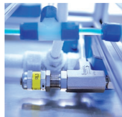
Pressure release valves are installed as safety precautions
